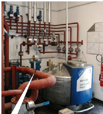
Figure 4.27: Pumping station number 2 with a filter and a waste container for cleaning the filter [50, Germany, 2006], [51, EuLA, 2006]
