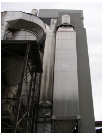
Figure 1.66: Example of an SCR installation [140, Italy, 2007]
