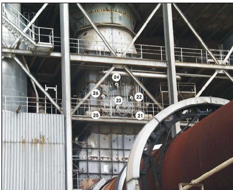
Figure 4.8: High efficiency SNCR and place for injection of ammonia water via lances at places Nr. 21 to 26 [76, Germany, 2006]
