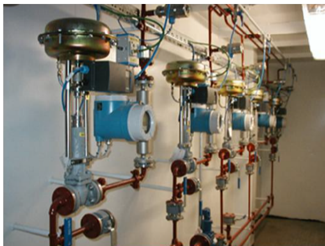
Figure 4.28: Measuring and dosing station with pneumatic valves [50, Germany, 2006], [51, EuLA, 2006]
