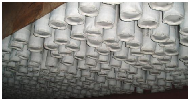
Figure 1.60: Example of a fabric filter and filter material used in a cement plant in the UK [82, CEMEX Rugby UK, 2006]
